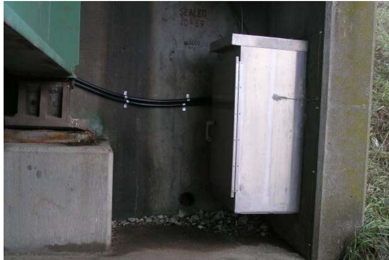
(a) Aluminum cabinet mounted on the north corner of the west abutment wing wall
